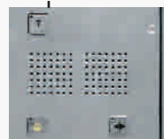
Controls embedded into the wall.
